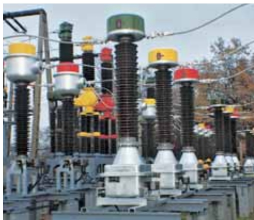
1. 123 kV Inductive voltage transformers (Bosnia).
