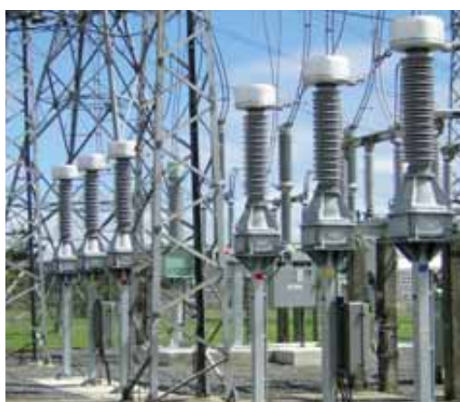
2. 123 kV Inductive voltage transformers. Transpower (New Zealand).
