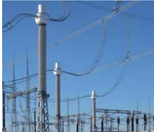
1. 765 kV Current transformer. RAO-FSK (Russia).
