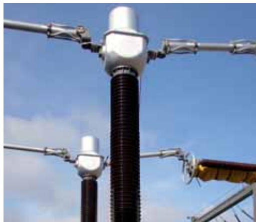
3. 420 kV Current transformers. National Grid (UK).
