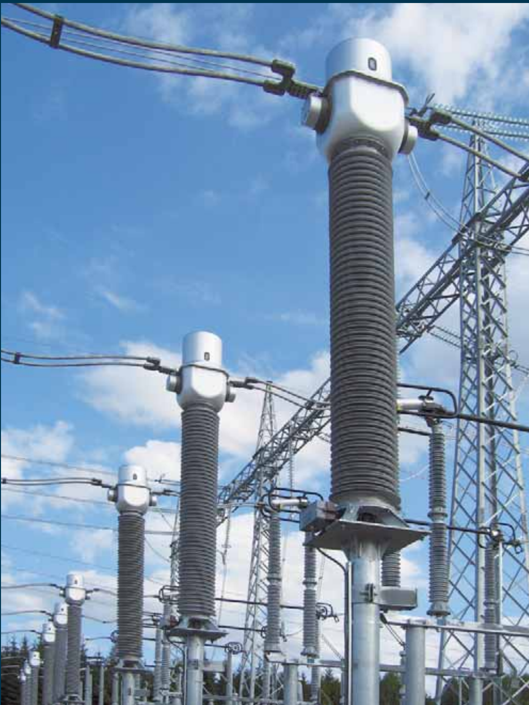
> 420 kV Current transformers with gray silicone rubber insulator. Statnett (Norway).
