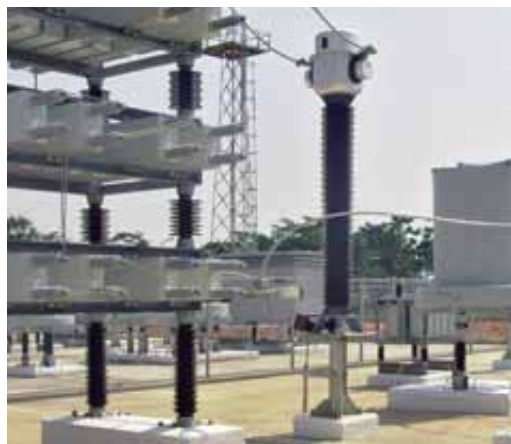
2. 245 kV Current transformer protecting capacitor bank (India).
